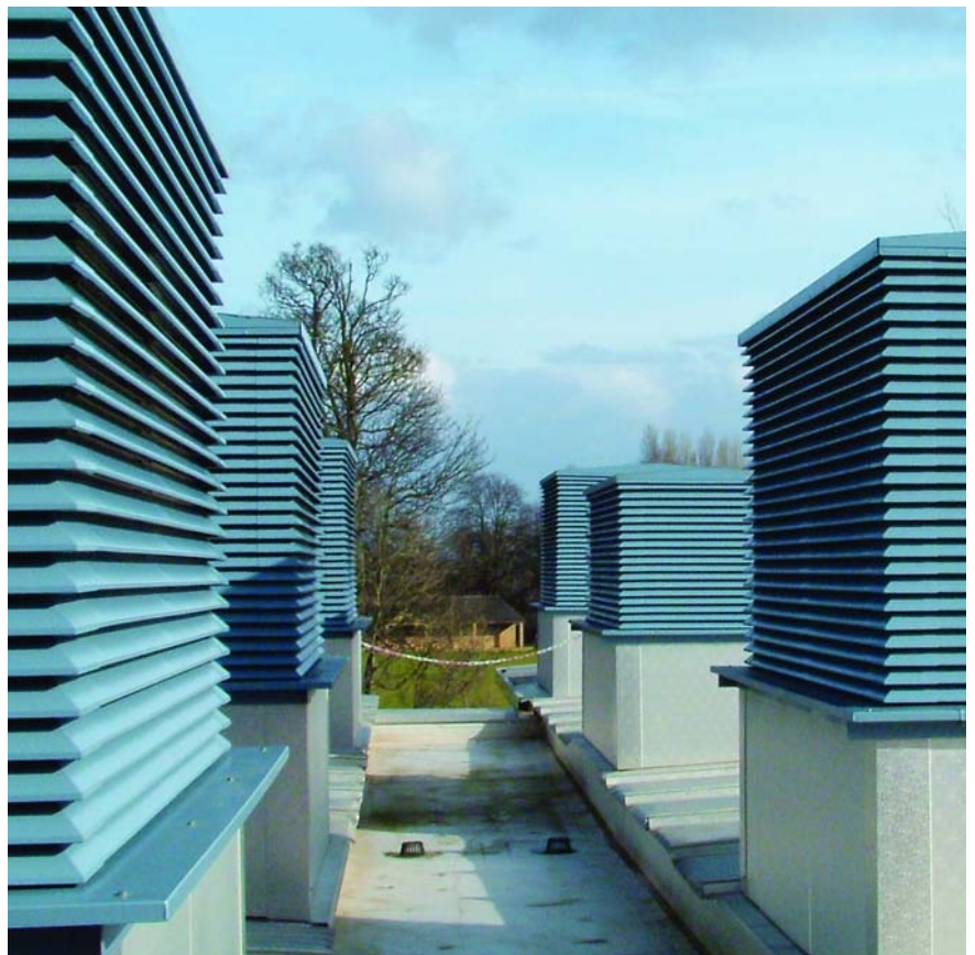
Portway School, Bristol Pre-assembled 3UL louvre turrets on top of natural vent shafts.
