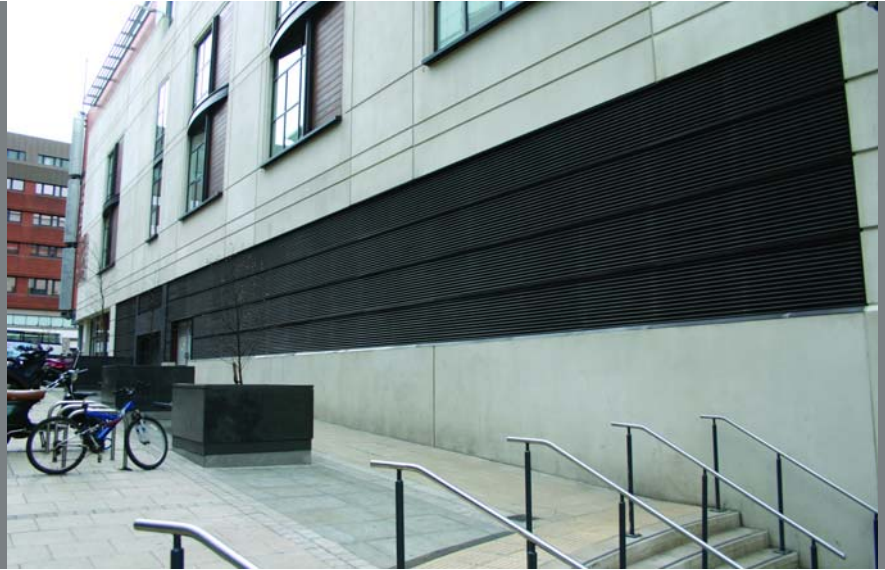
The Light, Leeds. Single bank 1UL louvre upgraded to 3UL for "live" areas.
