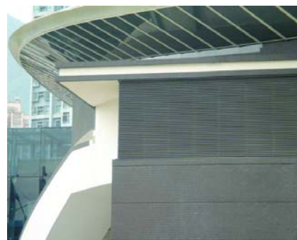
Indoor Recreation Centre, Ma On Shan, Hong Kong. Universal Louvre for plant room ventilation and for controllable air inlet for the smoke extraction system.
