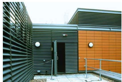
Evelina's Childrens' Hospital, London. Plant room louvres and doors.
