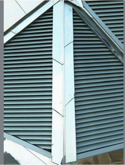
C-Plex, West Bromwich. Trapezoidal 2UL louvre panels.
